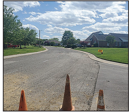
Figure 2: Typical Milled out Roadway
