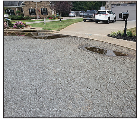
Figure 4: Severe Alligator Cracking/Rutting
